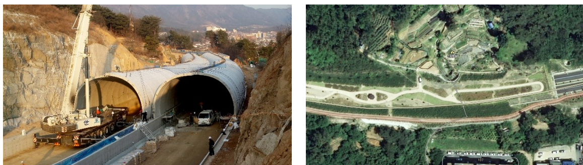
Fig. 6 Precast arch tunnel adjacent to a steep rock incision in urban area
