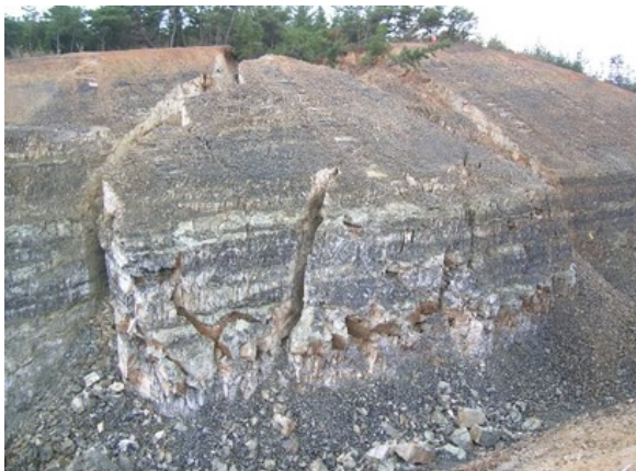
Fig. 7 Rock slope collapsed due to the blasting vibration
